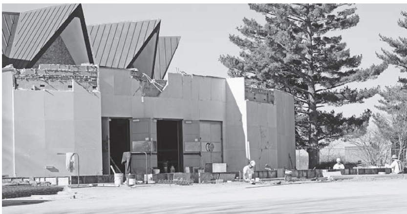
Construction workers from Sircal Contracting Inc. work on laying the foundations for an enlarged gathering space, known as a narthex, and sinking the shaft for an elevator to the Undercroft as part of major renovations to the Cathedral of St. Joseph in Jefferson City.
